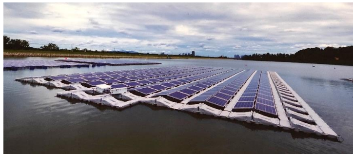
Figure S5. Floating photovoltaic system at Singapore's Tengeh reservoir.
