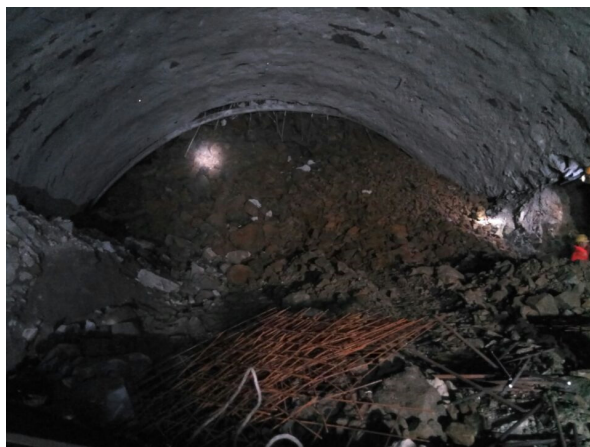
Figure 2. Collapse in the section DK229 + 671~ DK229 + 725 of Huangjiazhuang tunnel.
