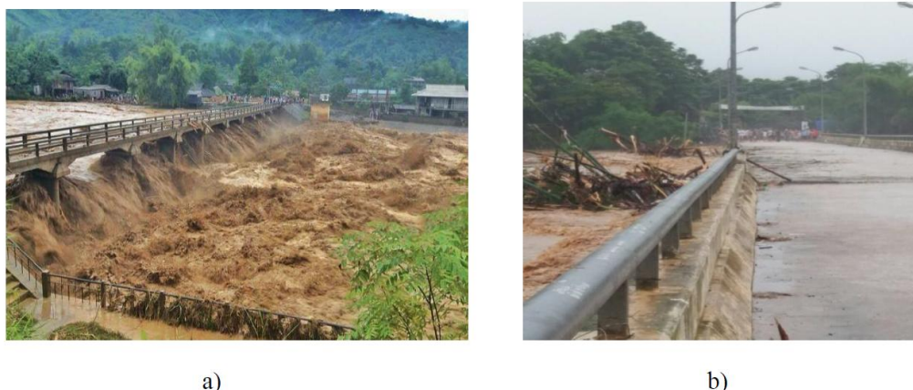
Figure 1. Examples of bridge pressure flows: a) Nghia Lo bridge in Yen Bai, Viet Nam, was partially inundated after heavy rains in 2017; b) Canh Nang bridge in Thanh Hoa, Viet Nam, was partially inundated under dam-break flow in 2018.
