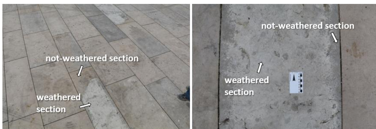
Figure 2. Outdoor pavement in “blue” limestone with visible alteration.
