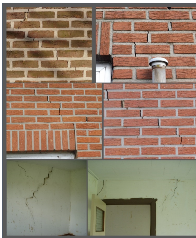
Figure 2. Some examples of post-mining induced damage in masonry during the uplift phase. All examples are situated within the study area of this paper (coal mine of Eisden, Belgium).
