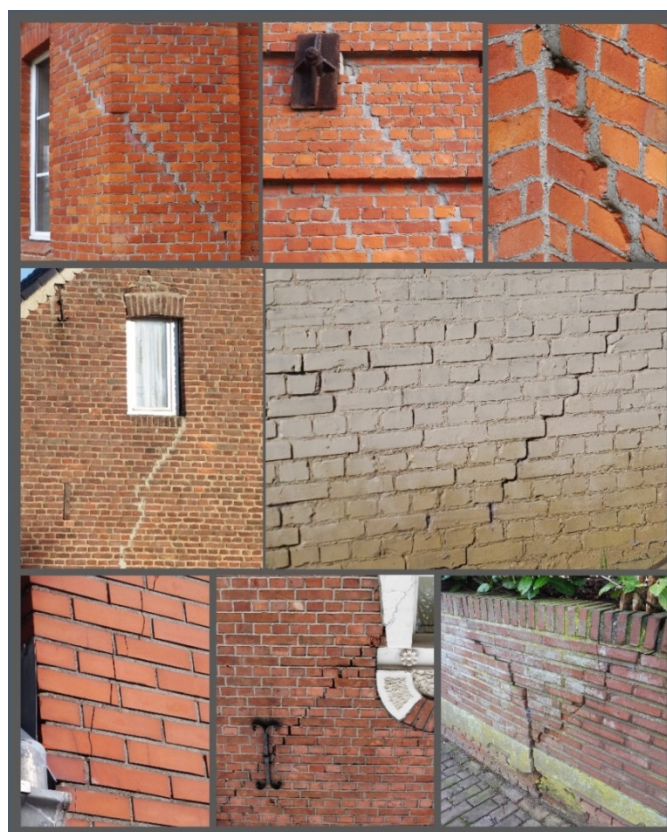
Figure 1. Some examples in the Campine coal district, Belgium of mining induced damage in masonry during the subsidence phase.
