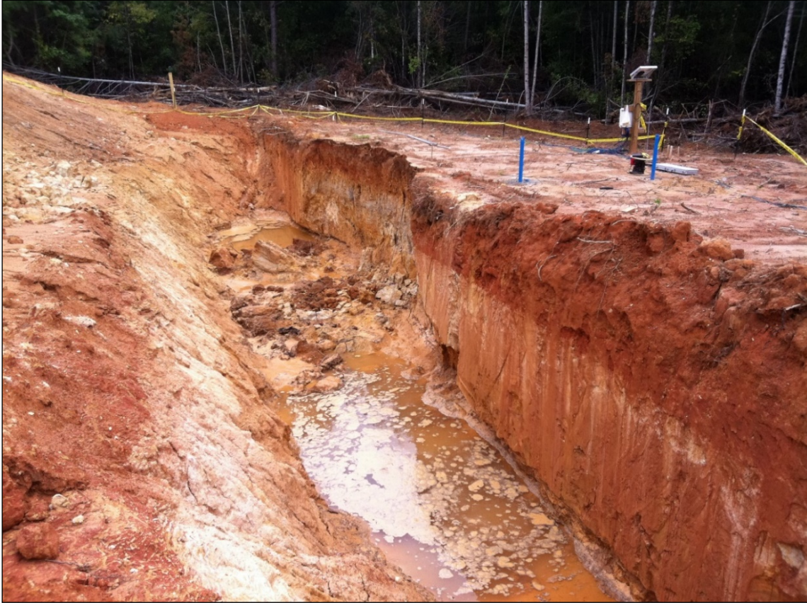
Figure 10. Excavation #2 after initial failure on 9/21/11.
