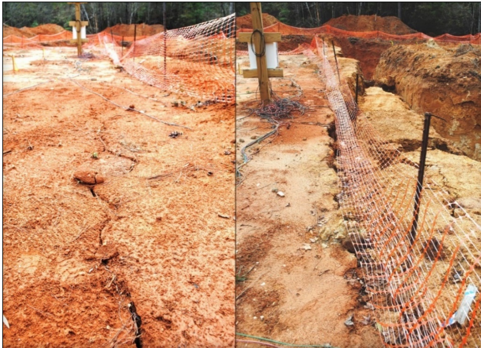
Figure 11. Tension crack progression over time (Excavation #1).
