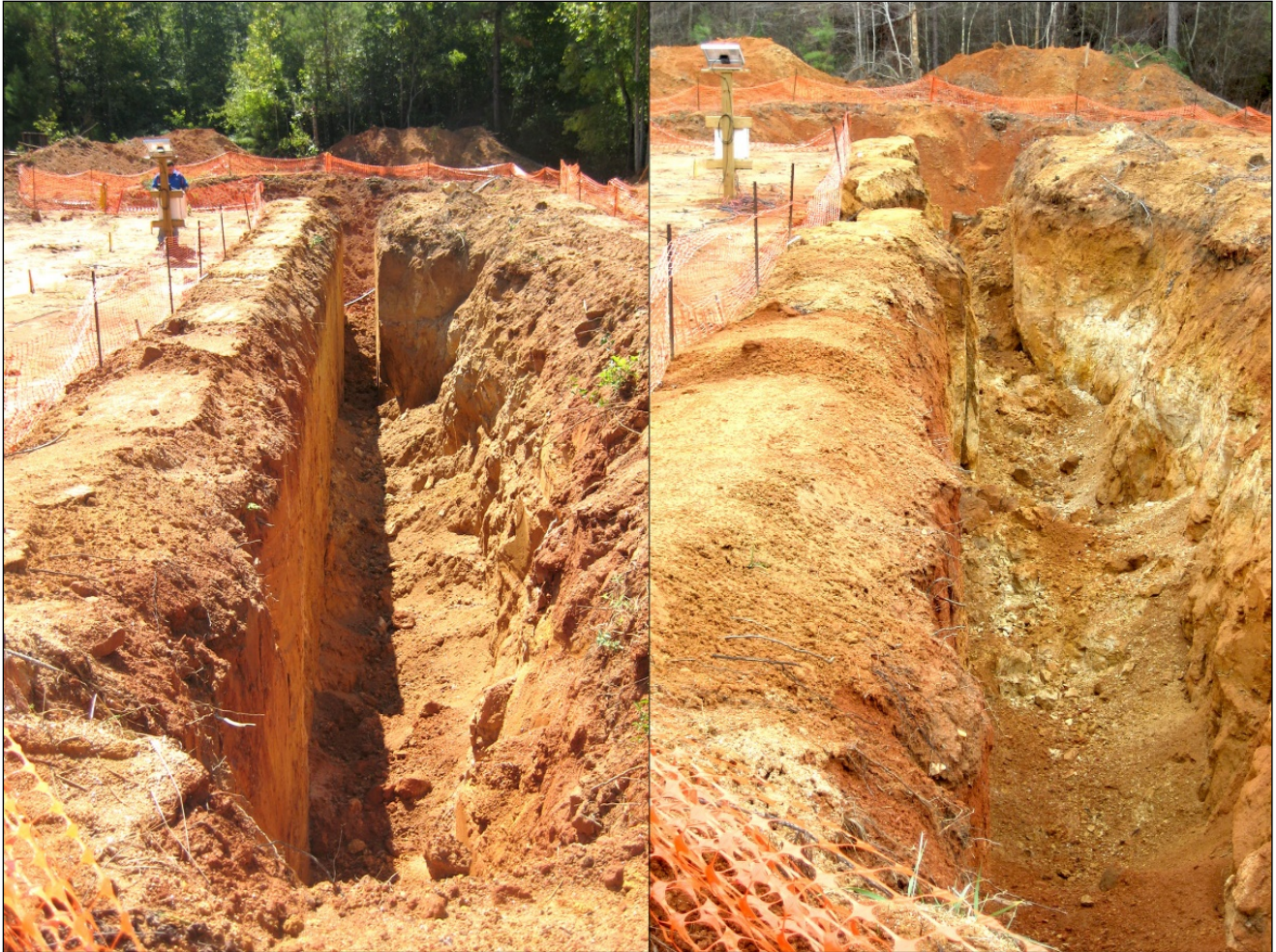
Figure 8. Excavation #1 before and after failure.
