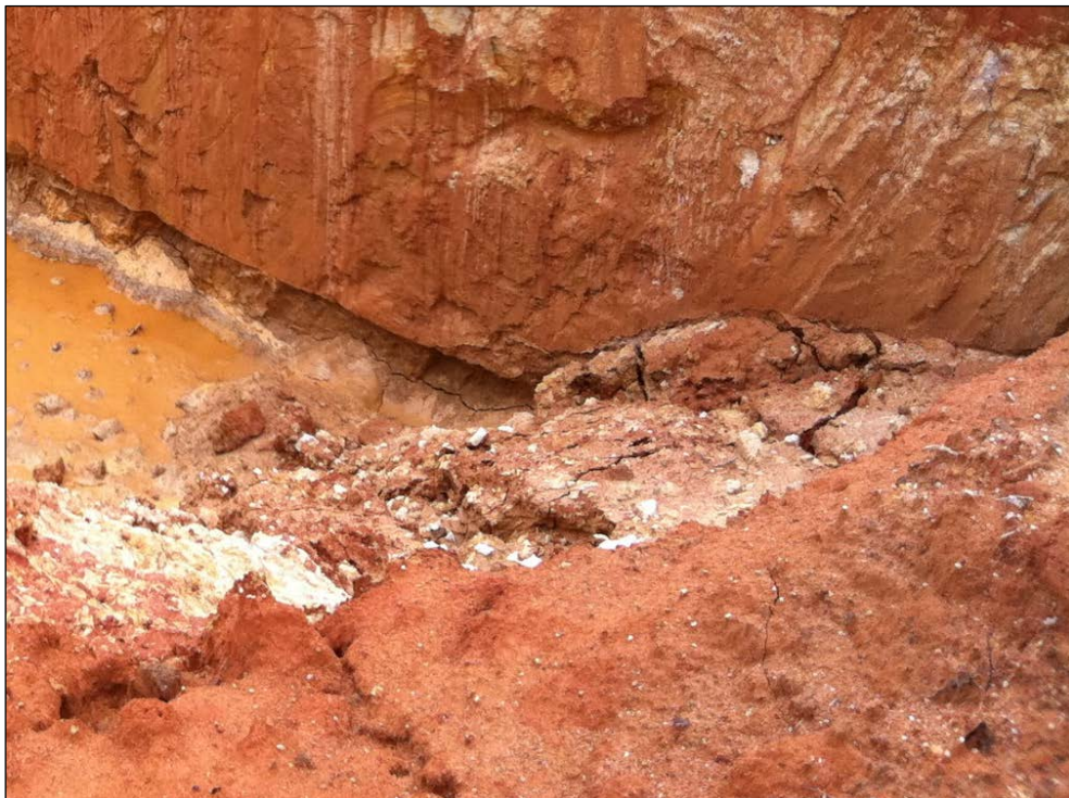
Figure 7. Undermining from water in bottom of trench.
