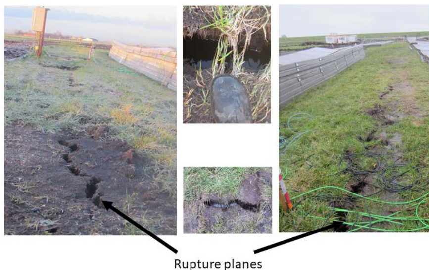
Figure 5. Typical rupture planes found on the active side of the failure plane.
