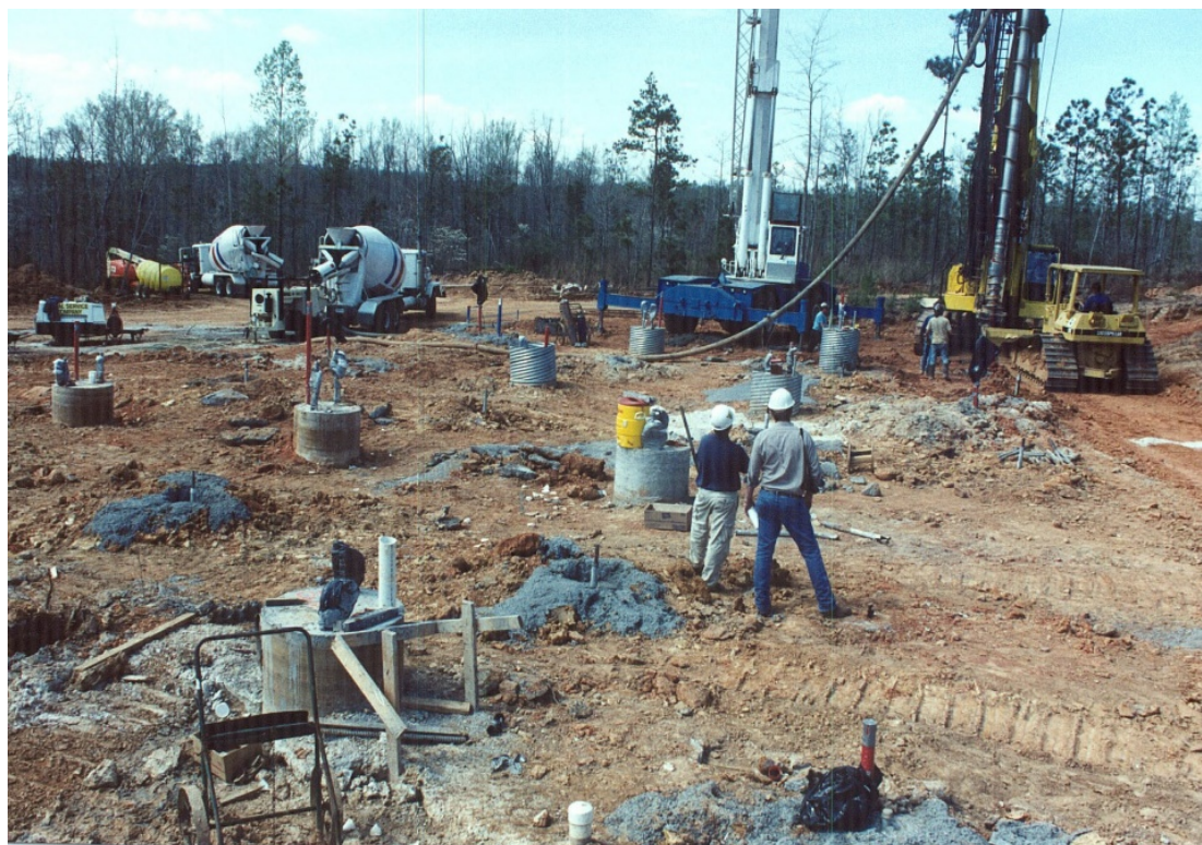
Figure 5. Installation of drilled shafts and displacement piles (photo courtesy of Dan Brown).
