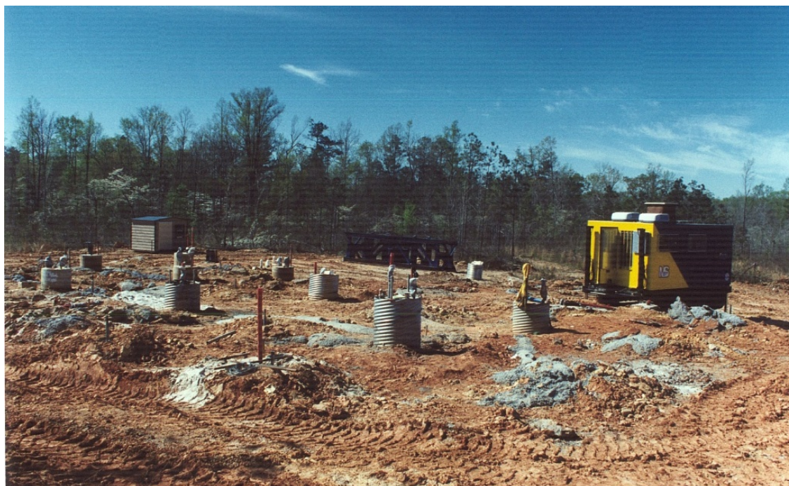
Figure 4. Early cone penetration testing at the AUNGES (photo courtesy of Dan Brown).
