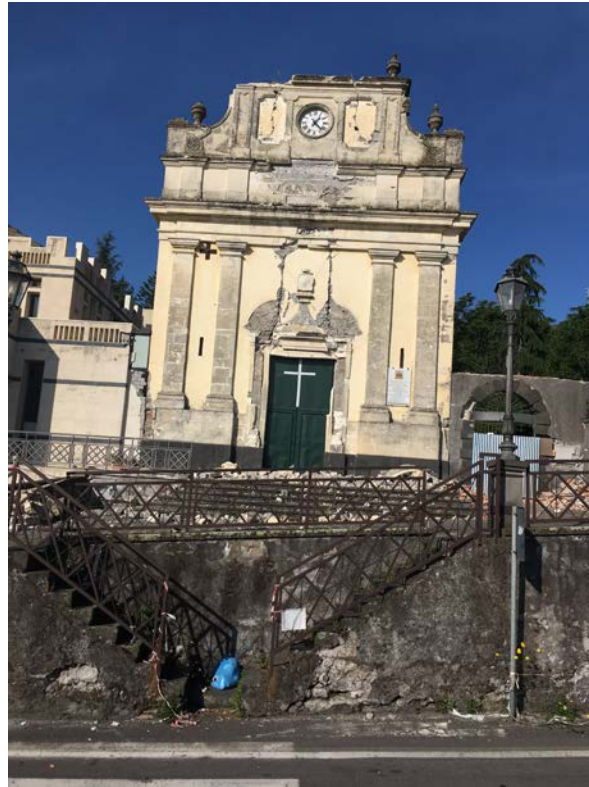
Figure 2. Church of Santa Maria del Rosario (Fleri) after the earthquake that occurred on December 2018. (Ph. Leonardo Mercatanti).
