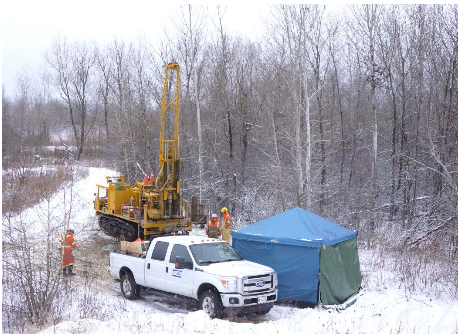
Figure 8. Setup and rig used for in-situ testing at Gloucester NRC-1 site, Ontario in 2014.
