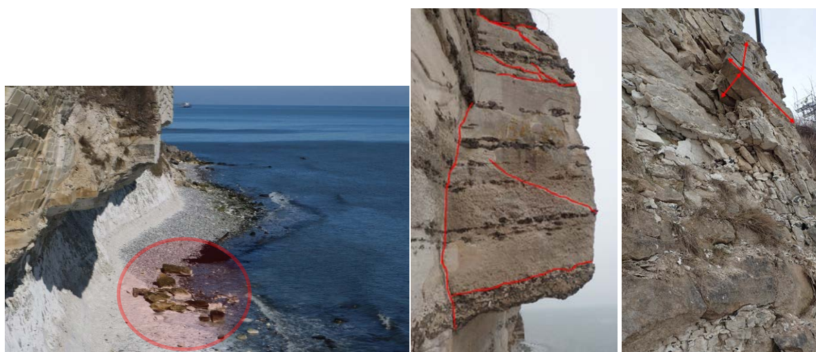
Figure 5. Overhang; rock fall and fractures on the slope (outlined with red; block group 40 \times 50 \times 150 \text{ cm}^3 of about 800 kg). Photo J. Korshøj.
