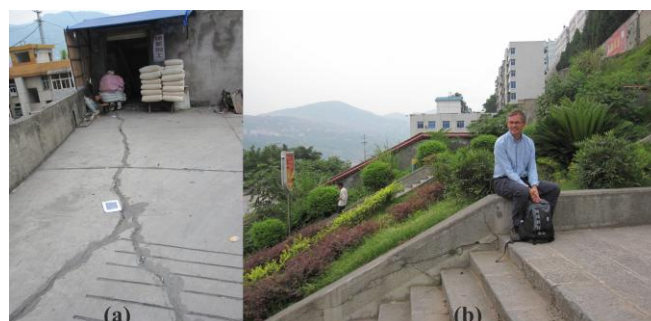
Figure 4. (a) A view of surface cracks seen in a landslide field in Badong County; (b) Surface displacements observed in a landslide field in Badong County.
