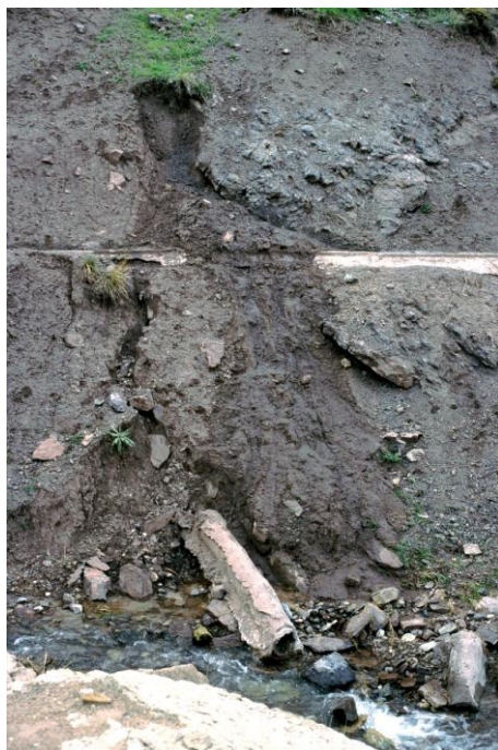
Figure 18. Water pipe damaged in research area (2002).
