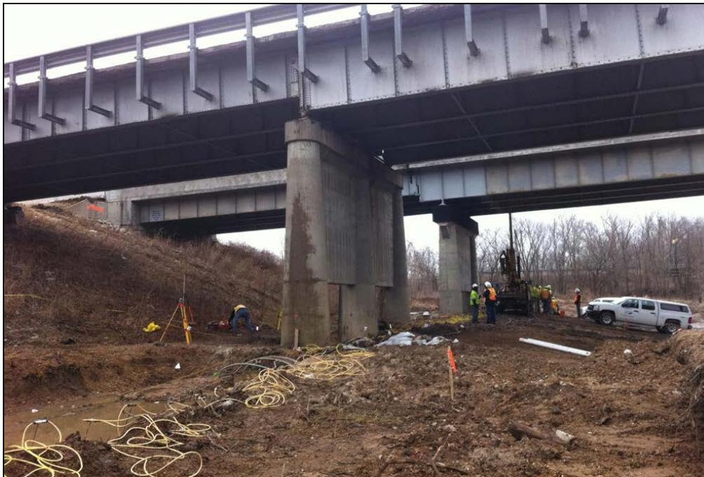
Figure 6. Photograph of the project site (looking southeast). ERT data are being acquired along Traverse 3.
