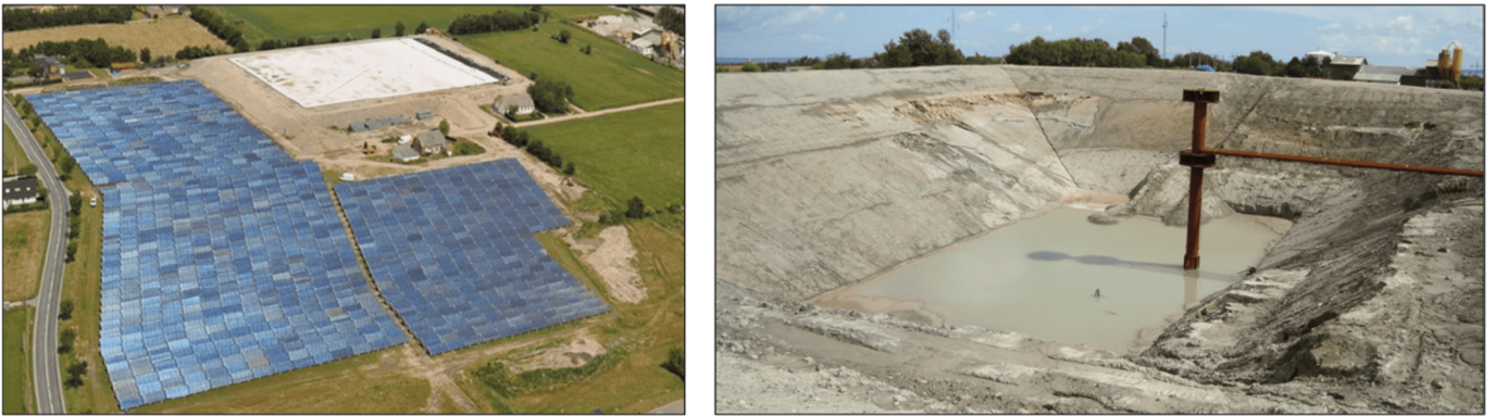
Figure 19. Aerial photo from 2013 (left) and diffuser installation in the PTES in Marstal (right) [163].
