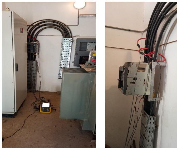
Figure 6. Three-phase power analyzer recorder installed at the main circuit breaker.
