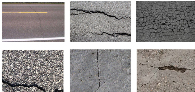
Figure 1. Examples of pavement crack.
