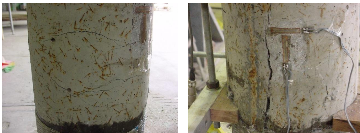
Figure 12. Cracking of corroded Hy-DFRCC column during structural test (left) and after failure (right).
