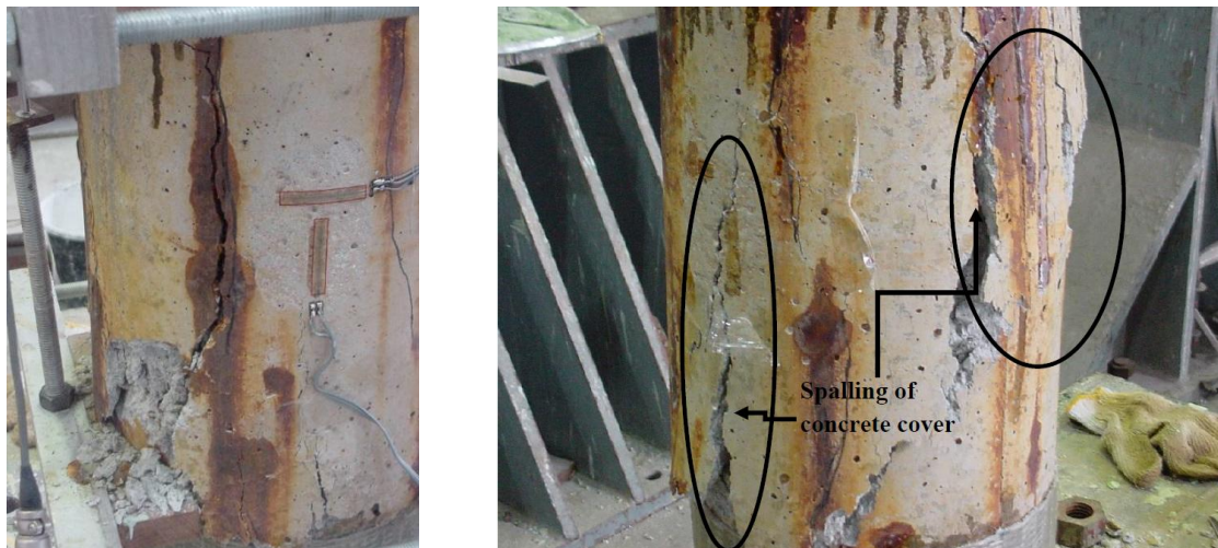
Figure 11. Spalling of clear cover of OPC-1 and OPC-2 corroded columns after failure load.
