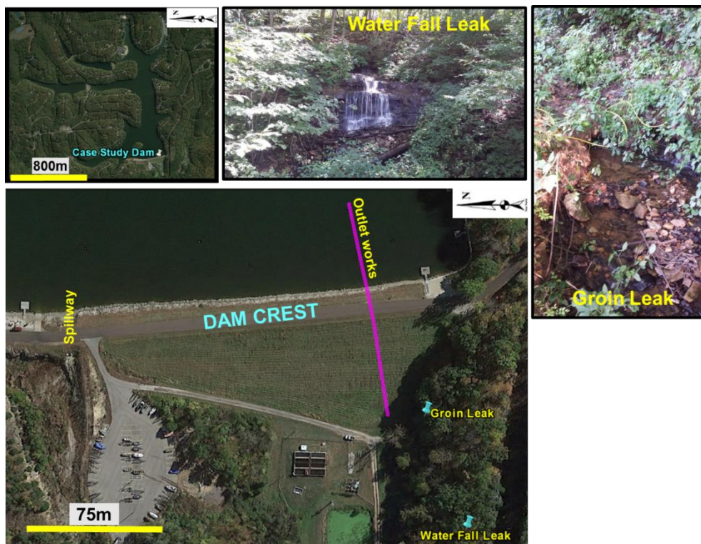
Figure 1: Approximate locations of the Groin Leak, Water Fall Leak and outlet works (drainage pipe).
