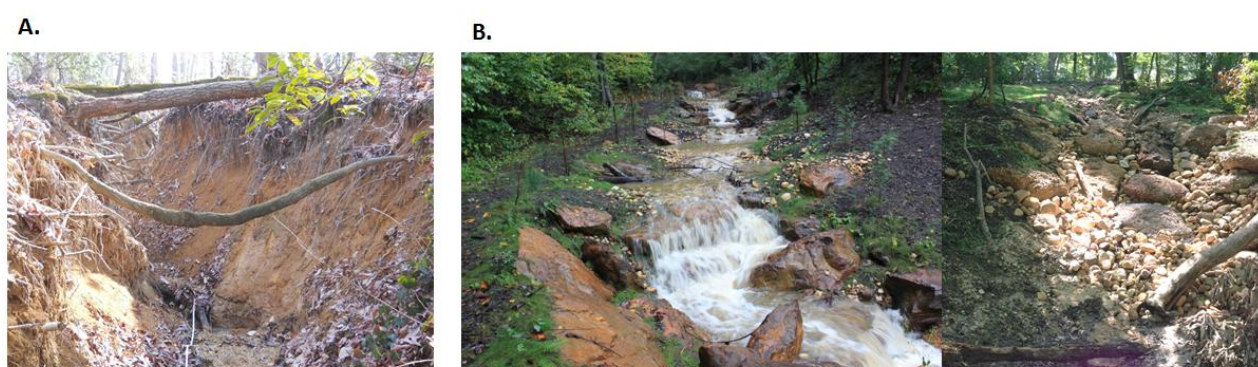
Figure 8. Example of (A) an eroded stream channel before; and (B) after a regenerative stormwater conveyance (RSC) restoration consisting of riffles, cobbles, and underlying sand seepage system.
