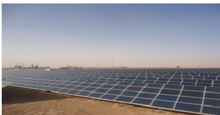
Figure 1. The solar photovoltaic station Kaberten-Adrar.
