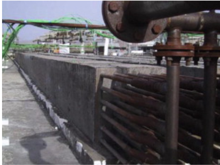
Figure 4. Thermal energy storage module (concrete) of solar platform in Almeria (Spain) [84].
