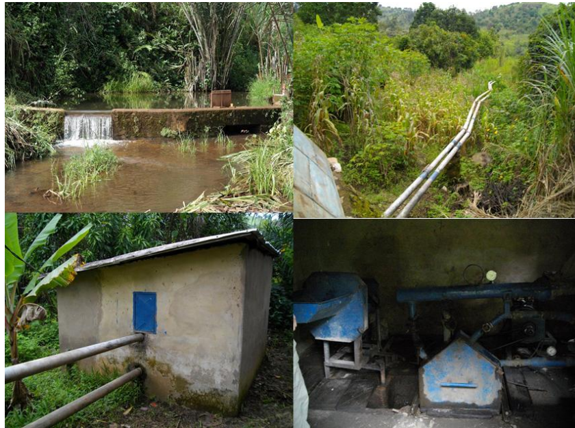
Figure 5. Component of the micro hydropower schemes; top left-Weir to divert part of the river into the intake; top right-penstock to convey water from the forebay to the powerhouse; bottom-left- power house; bottom right- turbine-generator set in the powerhouse.
