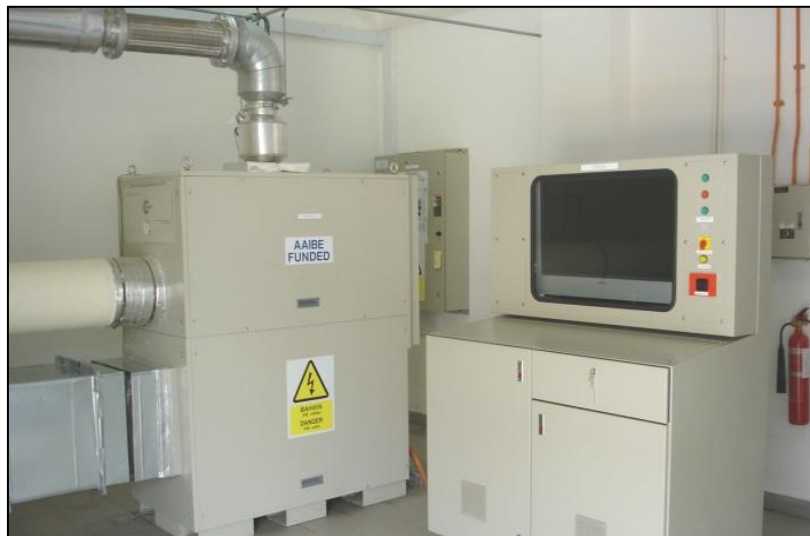
Figure 2. Oil fired microturbine system equipped with a data acquisition system.
