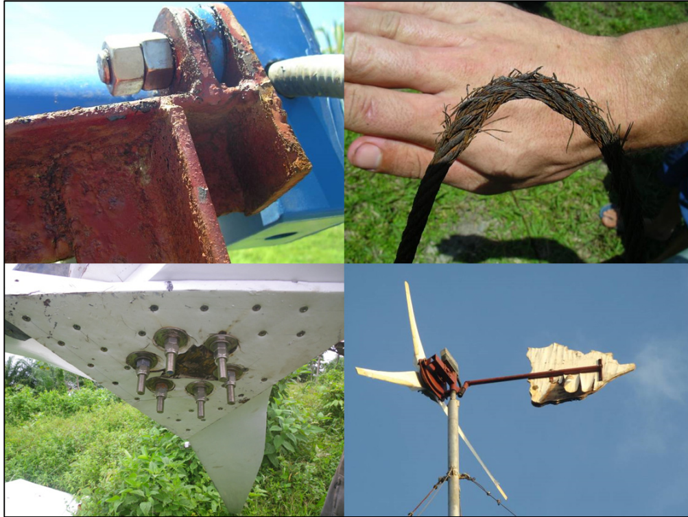
Figure 7. Different damages to SWT—Clockwise from upper left corner: Corrosion of body, corrosion of guy wires, tail vane water absorption and blade assembly damaged by water.
